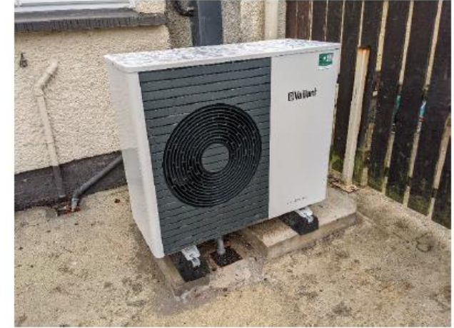
Vaillant Heat Pump as Part of Sunamp Installation
