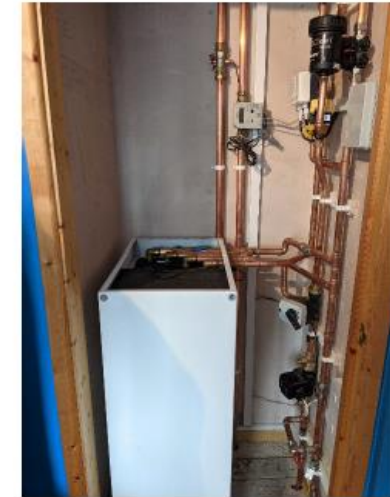
Sunamp Heating Battery Installation
